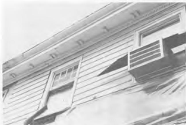
Detail of box cornice of the Williams Avenue house undergoing restoration; believed to be the former Planters Hotel.
