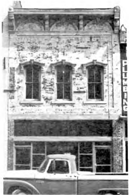
BEFORE: This two-story brick store house at 106 South Side Square was built in 1883 but through the years has suffered thoughtless modernizations and wanton neglect.
