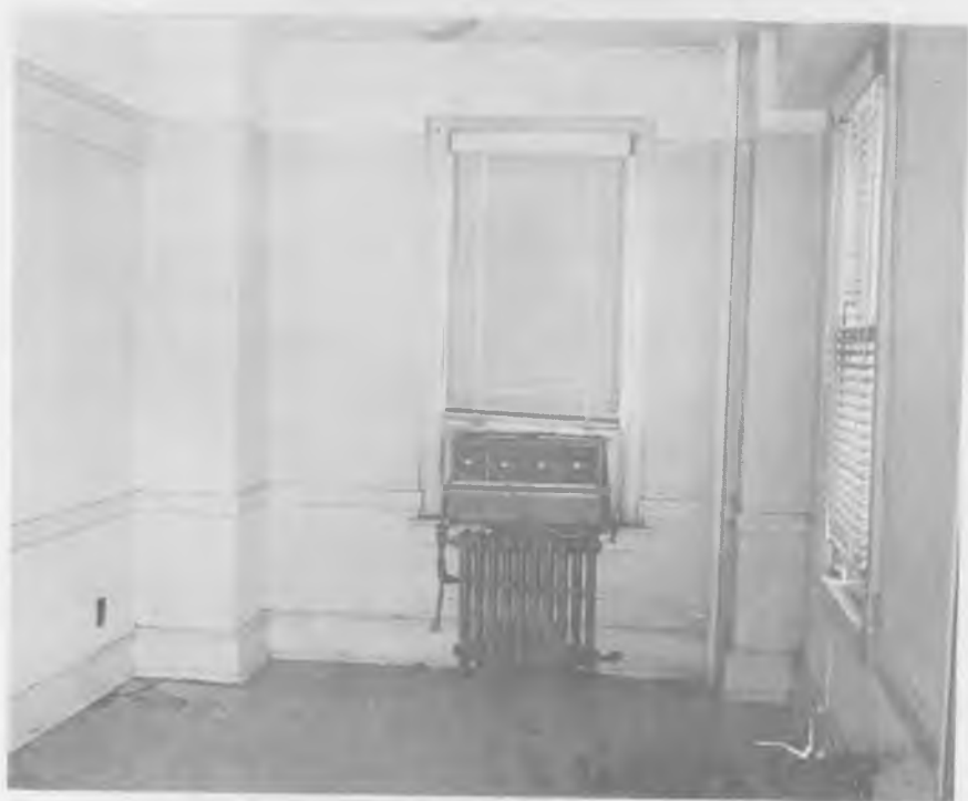
Notice the exposed plumbing for the radiator and how the concrete piers jut into the room.
