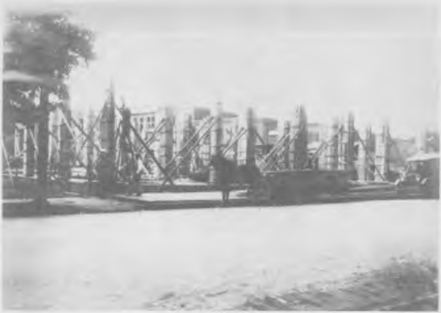
Construction of the Huntsville Daily Times building began in 1926 with the erection of wooden forms for the reinforced concrete columns of the first floor. Note the horse-drawn wagon at center.
