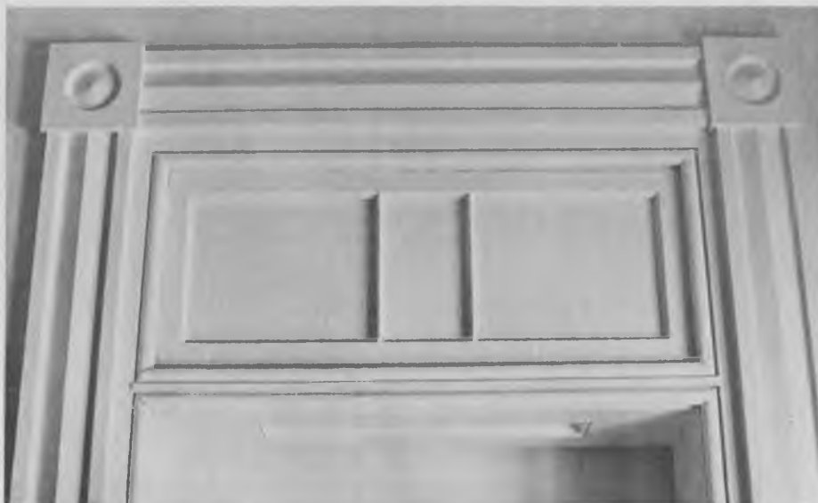
Interior doorway trim and transom in the entrance hall of OAK PLACE (ca. 1840) designed and built by architect George Steele for his own family. Steele was a leading proponent in Huntsville for the Greek Revival, as is evidenced by his designs for the second Madison County Courthouse, the First Alabama Bank, and Oak Place.
