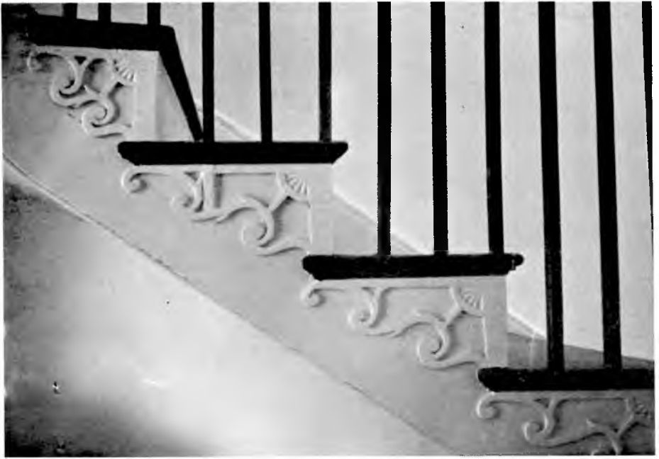
This detail of the stair scrolls shows how the pattern compresses as the stairway begins to curve.
