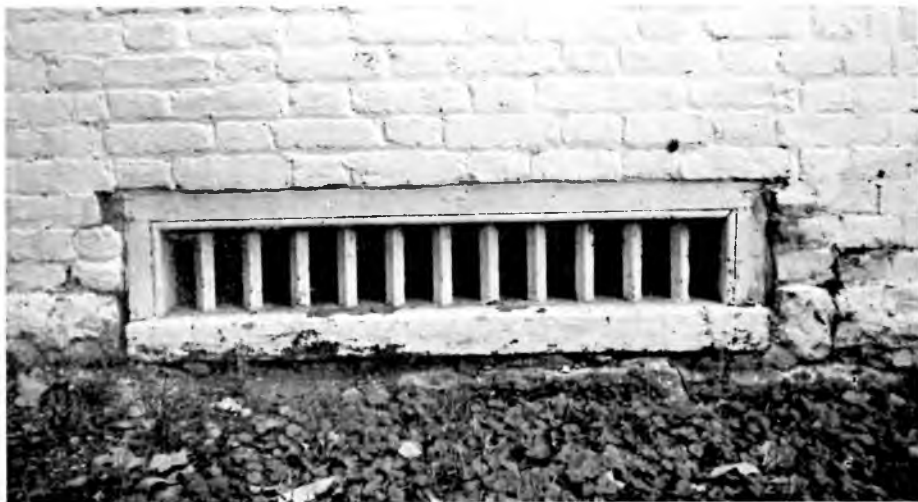
A foundation vent illustrating the diagonally placed bars and the three-quarter round mold framing the opening. Notice the Flemish bond of the surrounding brickwork.
