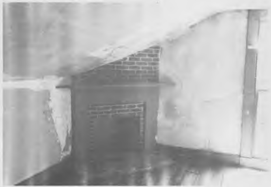
Corner fireplace in the unrestored east room upstairs. Note the sloping ceiling of the half-story level and the floor-to-ceiling length of the window.
