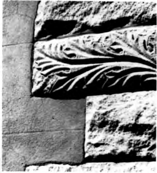
(12) Schiffman Building, 1895, side-entry stone arch. The fact that only the springer stones of the arch have foliated carving makes them seem more elegant than if all the stones were carved; an example of the power of contrast.
