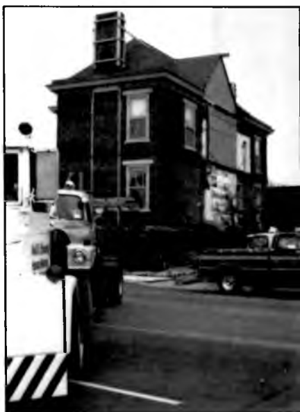
Pulling the house onto Monroe Street from its original site at Monroe Street and Clinton Avenue.
