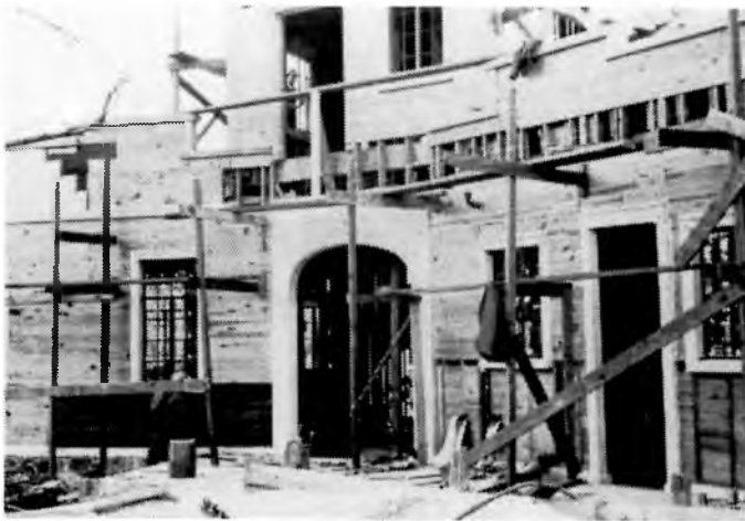
Construction of Burritt Mansion (2nd house), rear view before conservatory was added.
