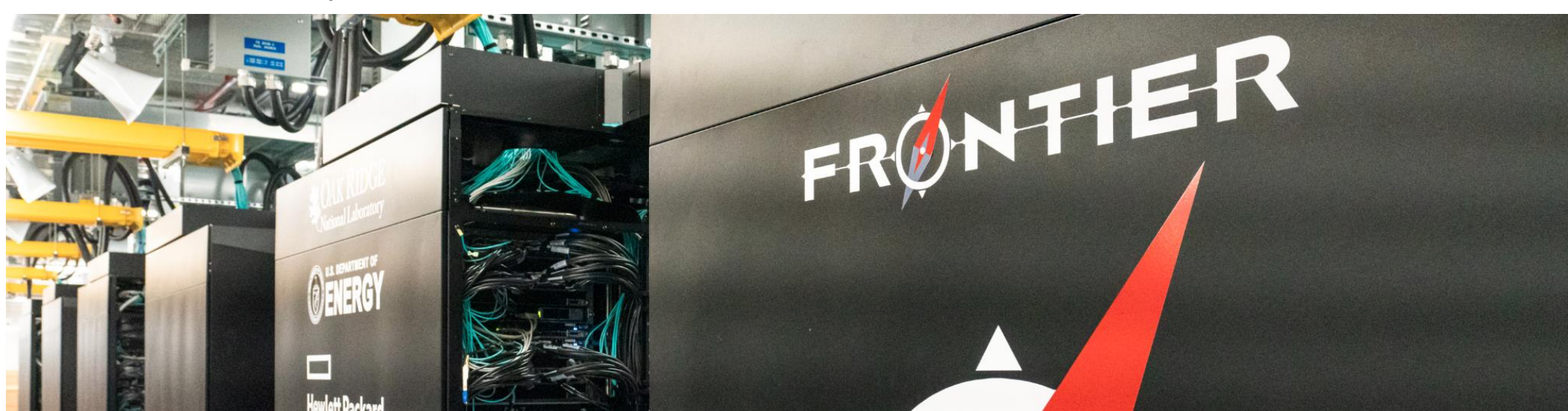
Pictured: Frontier, the world's first exascale supercomputer. Frontier will experience several faults every day due to its size and complexity.
