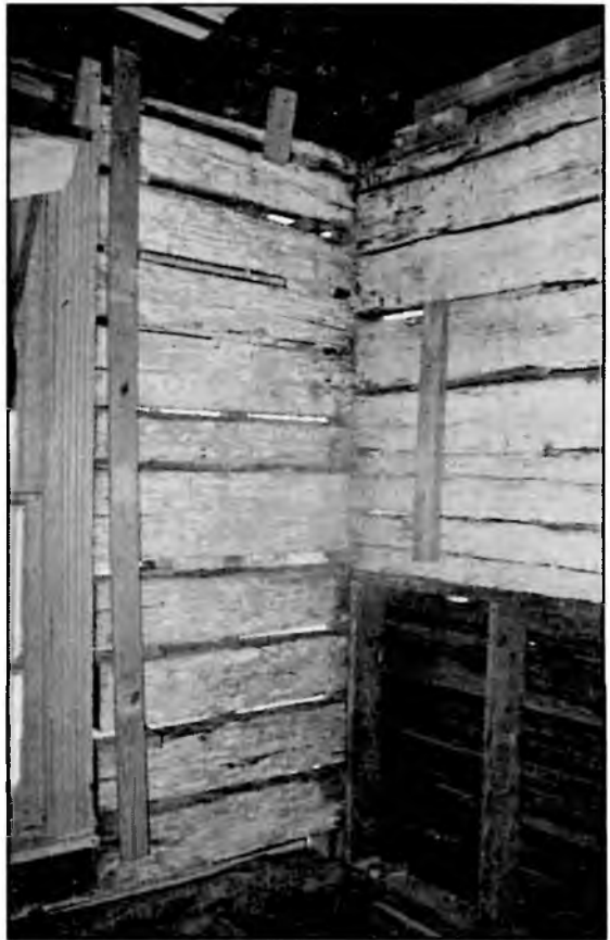
Fig. 6 Cabaniss-Ezell House, closeup of corner, repair in progress, late 1980s. Courtesy Gene Ezell.
