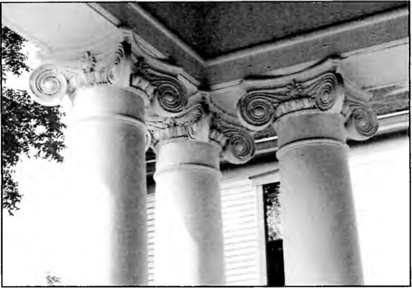
Fig.3 Detail on columns on porch of Johnson-Burwell Bungalow. Courtesy Jackson P. Burwell, P.C.
