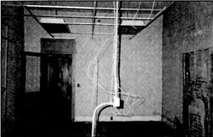
Fig.5 Drop ceiling frame and conduit Courtesy David Bowman
