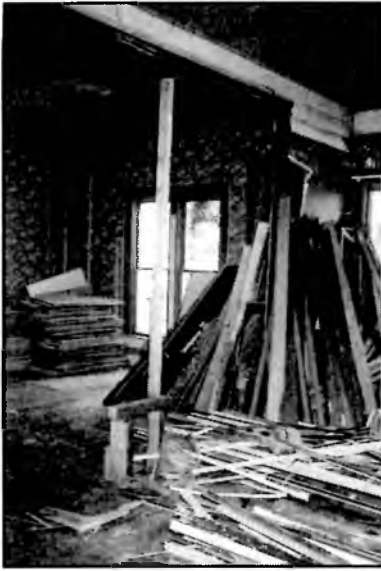
Fig.8 View showing deconstruction of interior of porch and room 4. Courtesy David Bowman.
