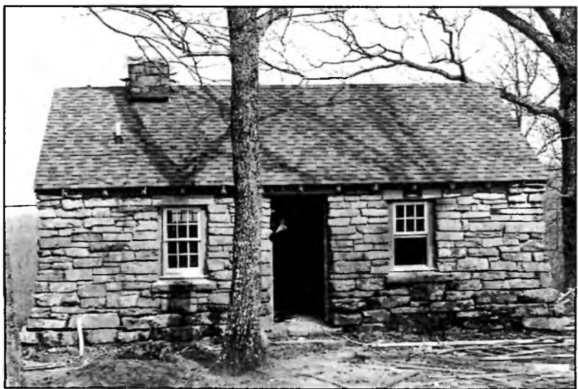
Fig.9 Cabin at Monte Sano State Park with new roof and new windows. Courtesy Kent Wilborn.
