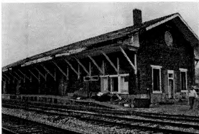
Fig.4 Track side and office end of freight depot, showing roof with shingles stripped off, October 1998.
