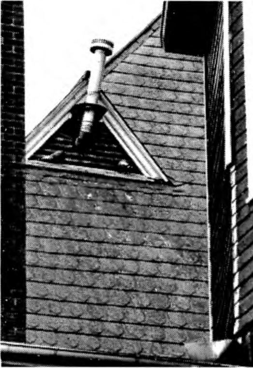
The Oscar Hundley House — Attic vent flanked by original brick chimney and 1930s elevator tower. Newer vent pipe intersects history and welcomes pigeons. Courtesy Harvie Jones Photo Collection.
