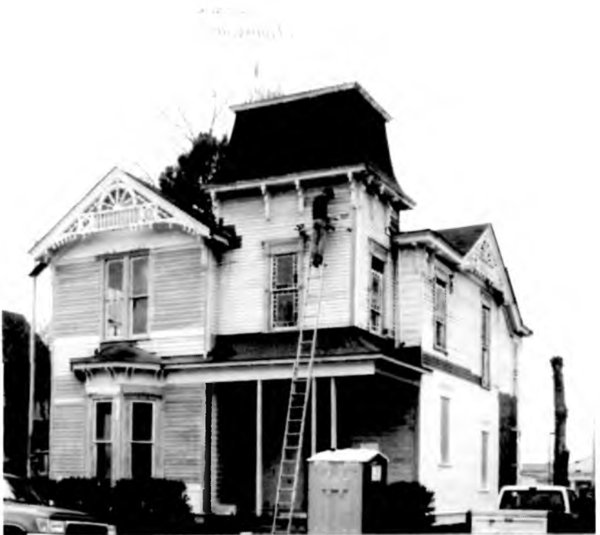
Figure 3: East front, Goldsmith-Donovan House, during restoration, December 1997. Joe Watson is atop the ladder:
