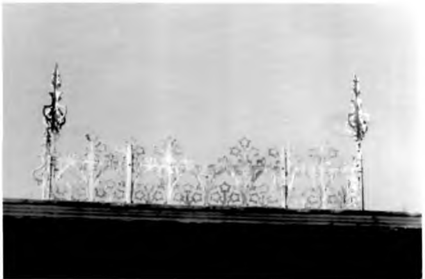
Figure 2: Metal cresting, tower. Goldsmith-Donovan House in 1996. Behind the finial at the right, a finial is missing.
