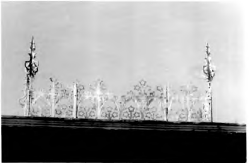
Figure 2: Metal cresting, tower. Goldsmith-Donovan House in 1996. Behind the finial at the right, a finial is missing.
