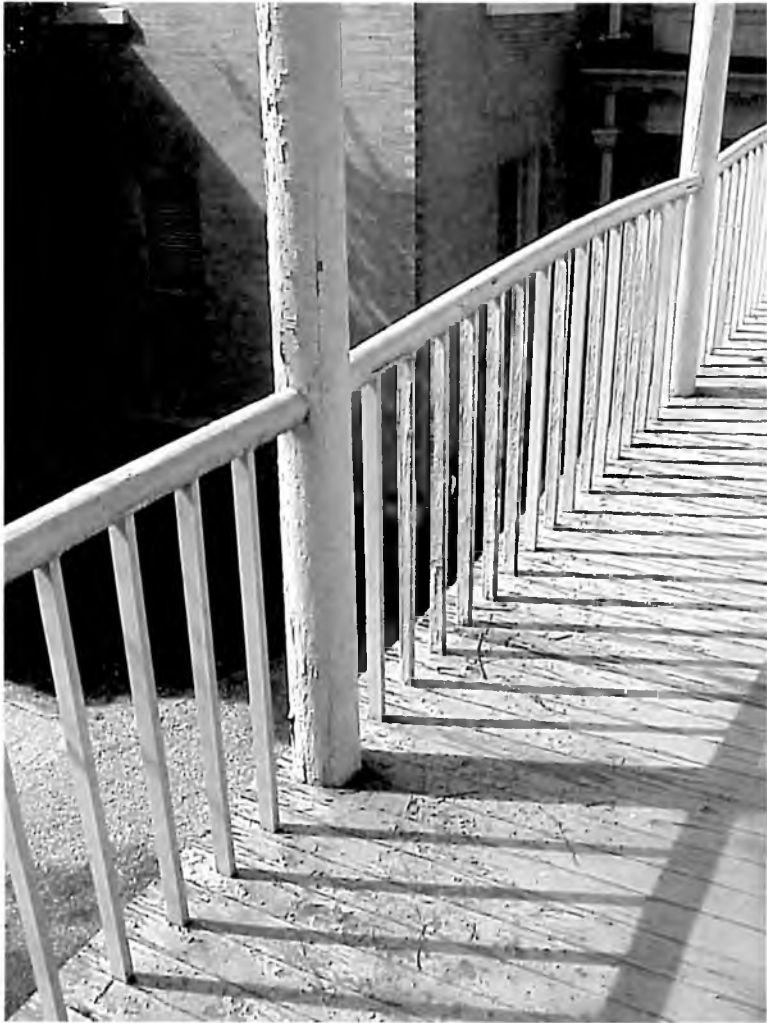
Detail of upper gallery railing. Elliptical profile handrail is intentionally cambered and is mortised into columns.
