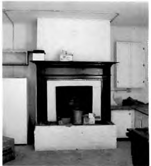
The only surviving mantel is in the lower level north room. The floor level of the room was lowered approximately 30 inches when it was converted to a garage.
