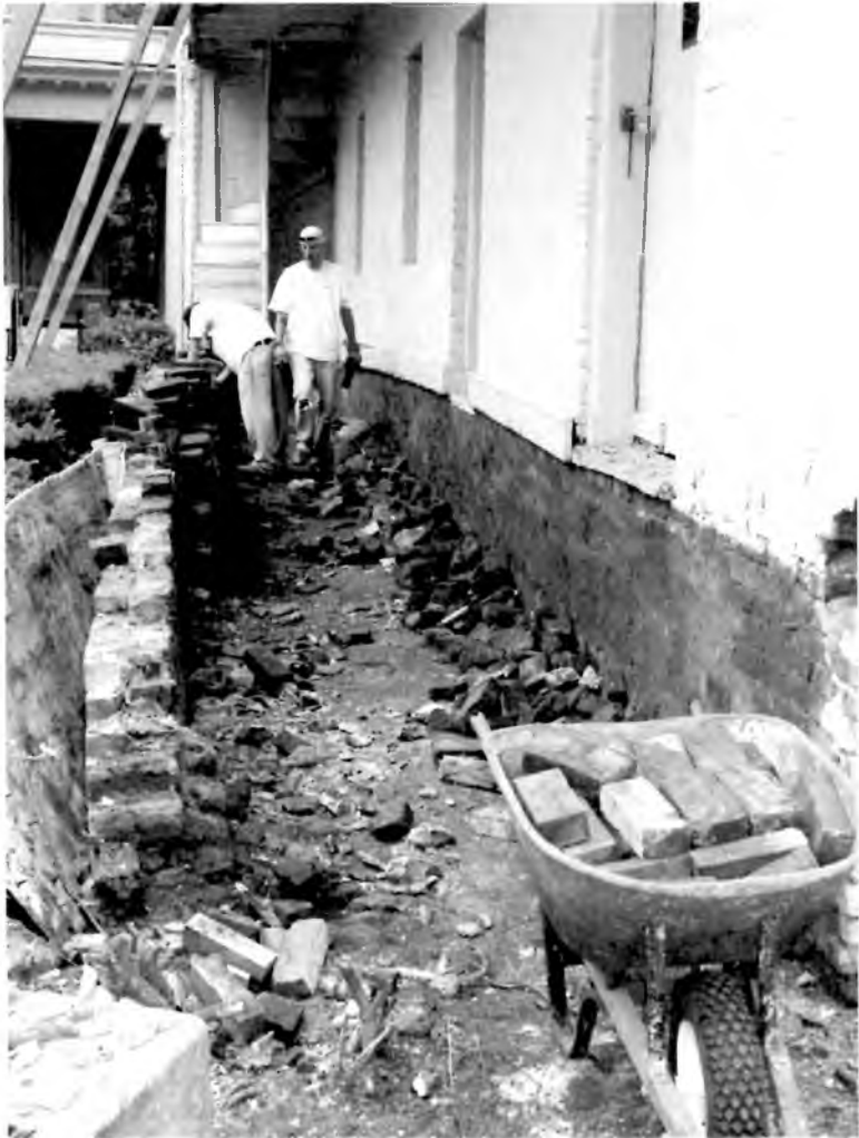
David Jones and Stacey Blazer of Wallace Construction discovered the site beneath the porch floor
