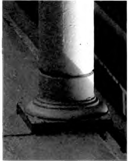
Detail of upper gallery column, modified Doric style capital with filleted neck
