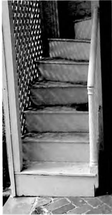
Detail of exterior stair at lower level gallery. Components appear to be re-assembled from previous construction.
