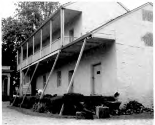
Restoration work begins on Lowe House outbuilding to shore up sagging porches
