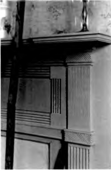
Detail of parlor mantel showing fluting and reeding. Photograph by Harvie Jones, F.A.I.A., 1981. Courtesy Architectural Collection of Harvie P. Jones, University of Alabama in Huntsville
