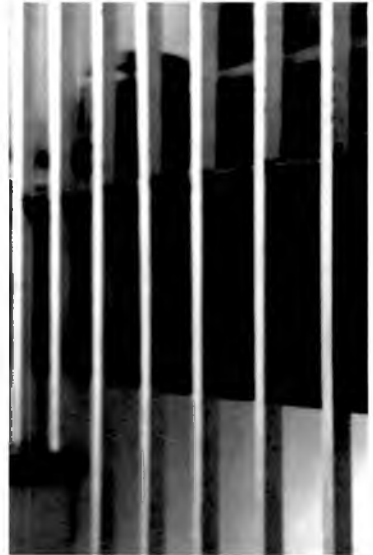
Landing balusters that pass through notches cut in the floorboard of the second-floor hall are an unusual feature. Photograph by Harvie Jones, F.A.I.A., 1981. Courtesy Architectural Collection of Harvie P. Jones, University of Alabama in Huntsville
