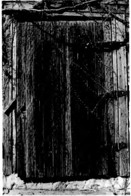
Batten door of Chapman-Johnson smokehouse. Smokehouse doors were often reinforced to deter unauthorized entry. The nail pattern seen here would have discouraged attempts to saw through the door. Photograph by Diane Ellis, 2006
