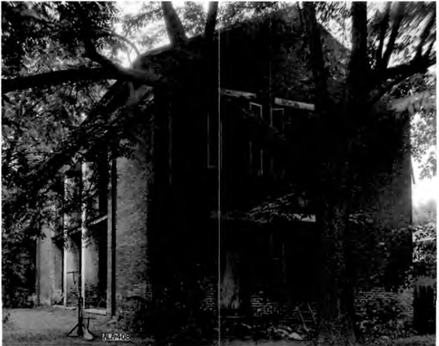
The north and east walls of the Lewis-Clay dependency show a major, two-story brick structure having inset galleries on both floors facing the back yard, supported by two-story, square brick columns. The scale, construction, and details indicate that this structure was intended to serve as more than a kitchen and servants' quarters. Demolished. Photograph by Alex Bush for HABS, 1935
