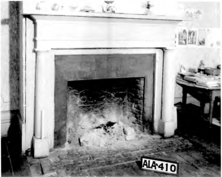
This fireplace protruded into the room and was more ornate, having an engaged column on either side. Faintly visible on the back wall of the firebox are bits of the design left by a cast iron fireback that was installed to help reflect heat into the room and protect the masonry of the chimney base. Photograph by Alex Bush for HABS, 1935
