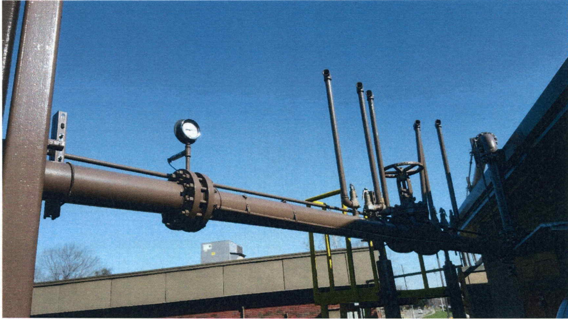
Figure 3.15: The analog and digital pressure gauges that measures pressure in the vertical supply tank, the six pressure relief valves, and the manual gate valve on the low-pressure piping system.
