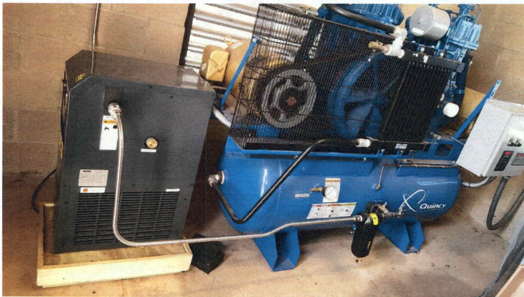
Figure 3.13: The air compressor and dryer used in the low-pressure piping system.
