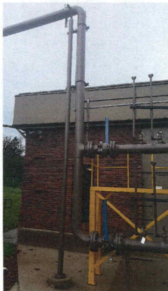
Figure 3.11: Piping system connection
