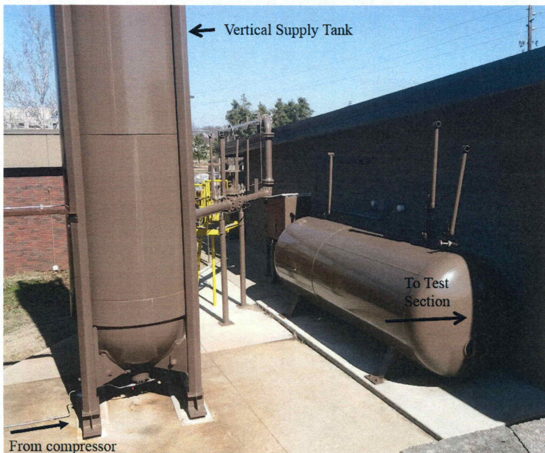
Figure 3.12: Photograph of the low-pressure piping system.
