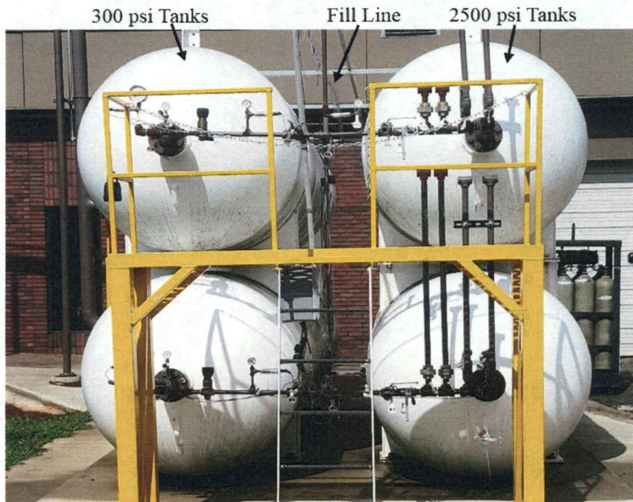
Figure 3.8: The piping and components connecting the 2500 psi tanks (right), the 300 psi tanks (left), and the fill line (vertical center).
