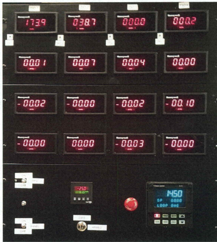
Figure 3.9. The control panel showing the digital displays for the pressure transducers.
