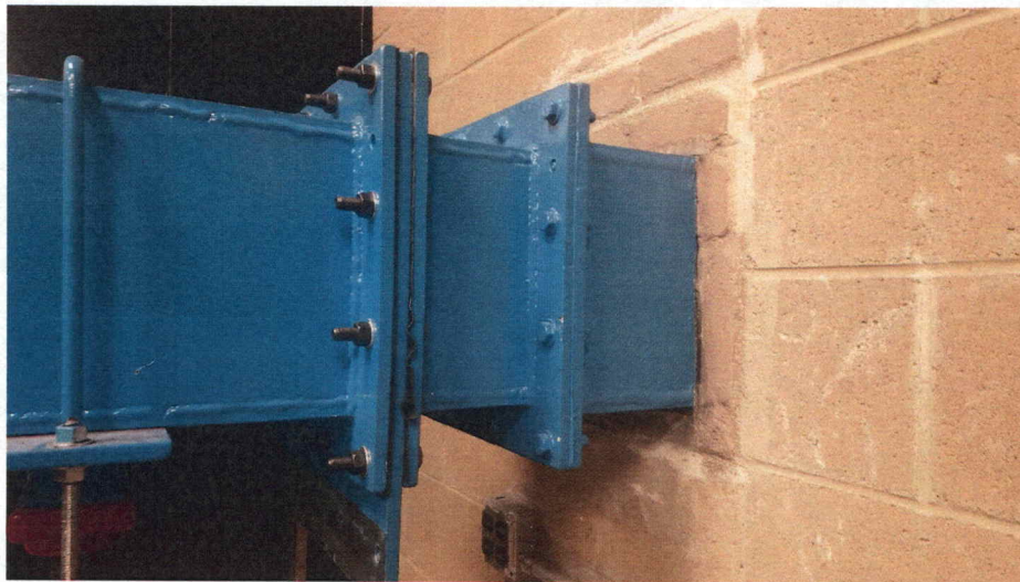
Figure 3.23. A photograph of the connection between the 10.635 inch duct and 9.635 inch square insert.
