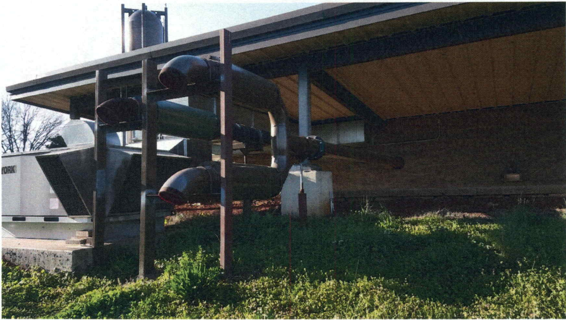
Figure 3.43: Exhaust piping for the wind tunnel facility.
