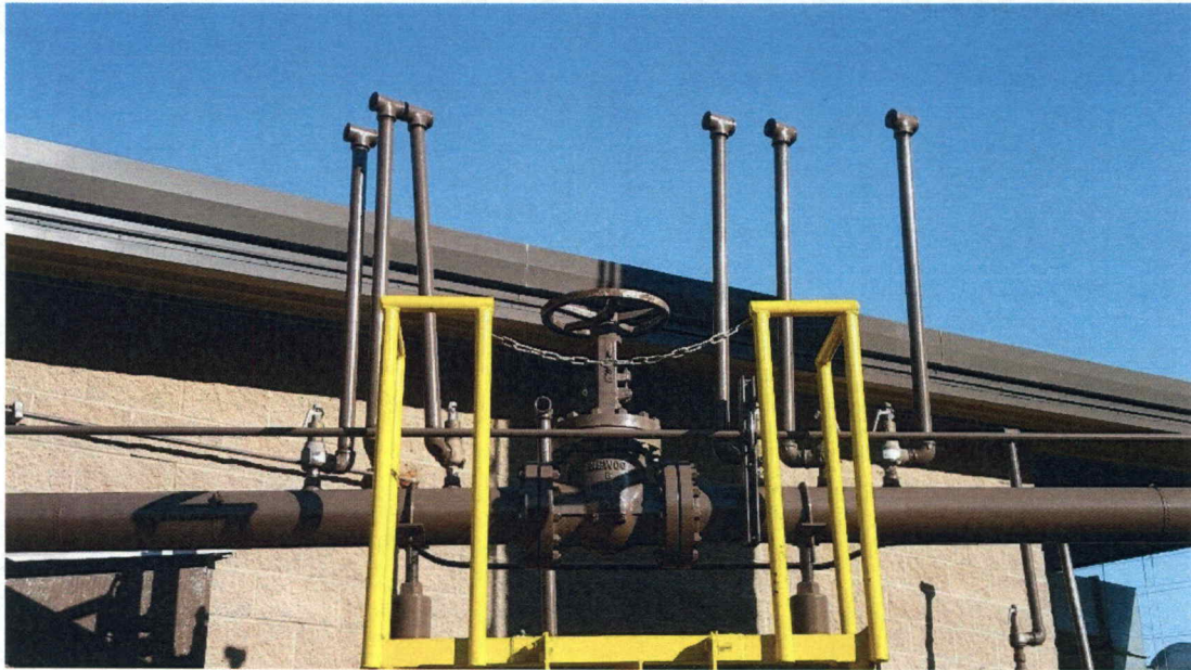
Figure 3.16: The six pressure relief valves and the manual gate valve on the low-pressure piping system.
